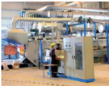
Pakistan Cables Nooriabad Factory (Pakistan)
